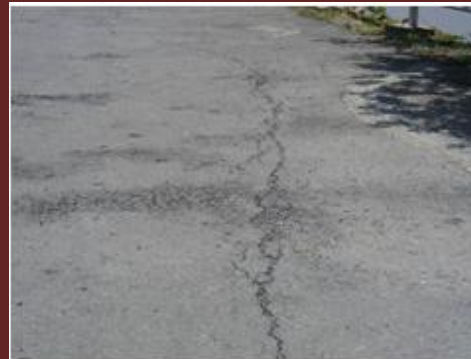
Crack on Dam Crest
